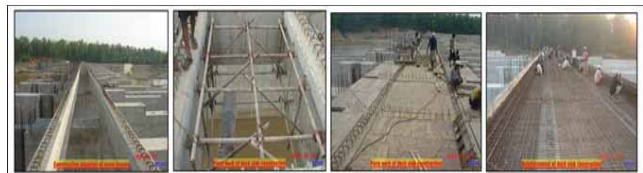
Fig. 3 Procedure for deck slab construction with precast girder as per method of statement
