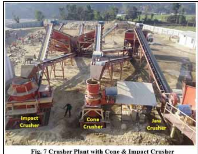
Fig. 7 Crusher Plant with Cone & Impact Crusher
