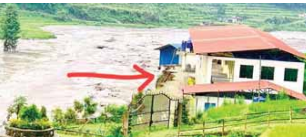
Figure 3- Bank cutting by the Helambu-Melamchi landslide flood
