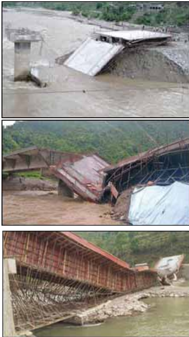
Fig. 4 Misguide of formworks design and procedure of deck slab construction
