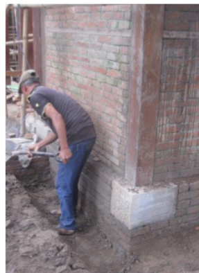
Up-rights (on I-Lohn) & Horizontal Ties for increased stiffness Of corner brick piers (2 nd Ring)
