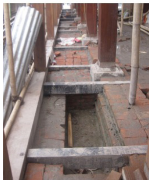
Tham with Lakasi & I-Lohn under – Suspended Floor (3 rd & 4 th Ring of Posts)
